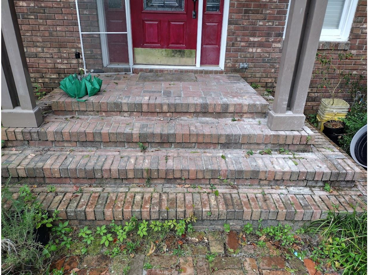
Thinset on brick porch, Photo 5.
