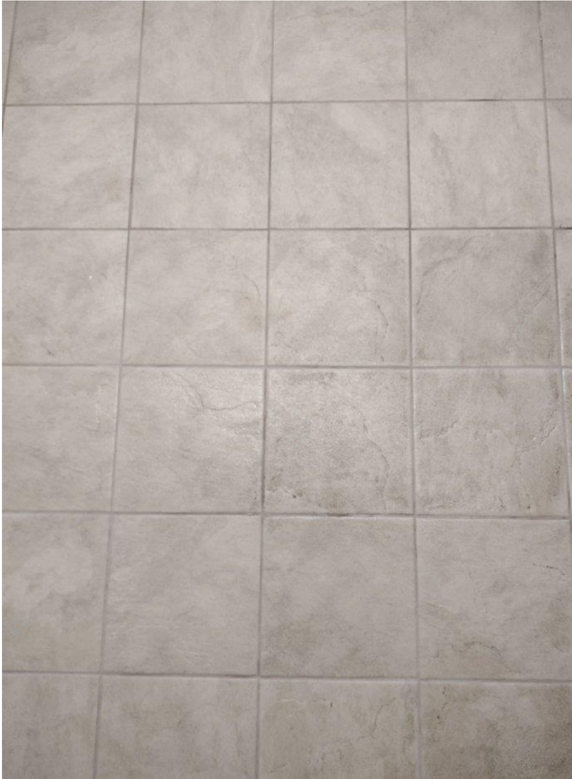
Grout cured on top of tiles, Photo 2. Grout cured on top of tiles for a permanently dirty look.
