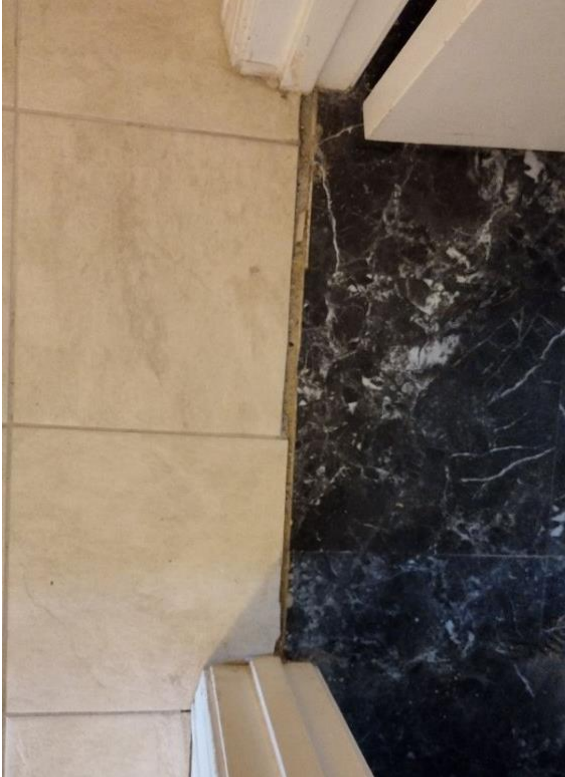
Jagged Edges, Photo 5. Finished threshold showing broken rather than cut tile edges.
