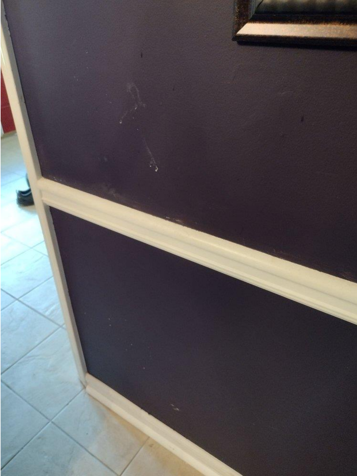
Grout on walls, Photo 7. Grout handprints on the walls.
