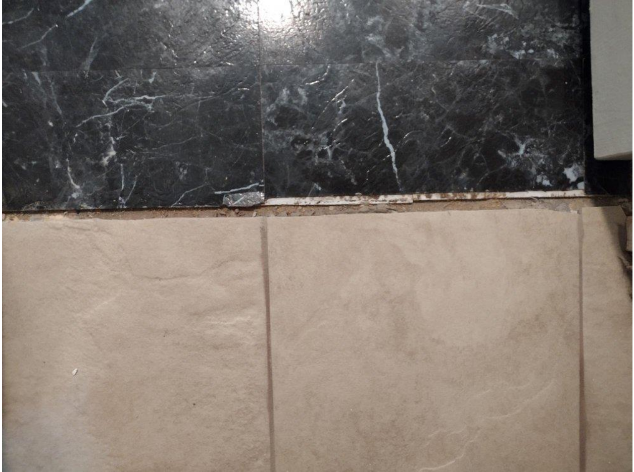
Jagged Edges, Photo 6. Finished threshold showing jagged edge of tile.
