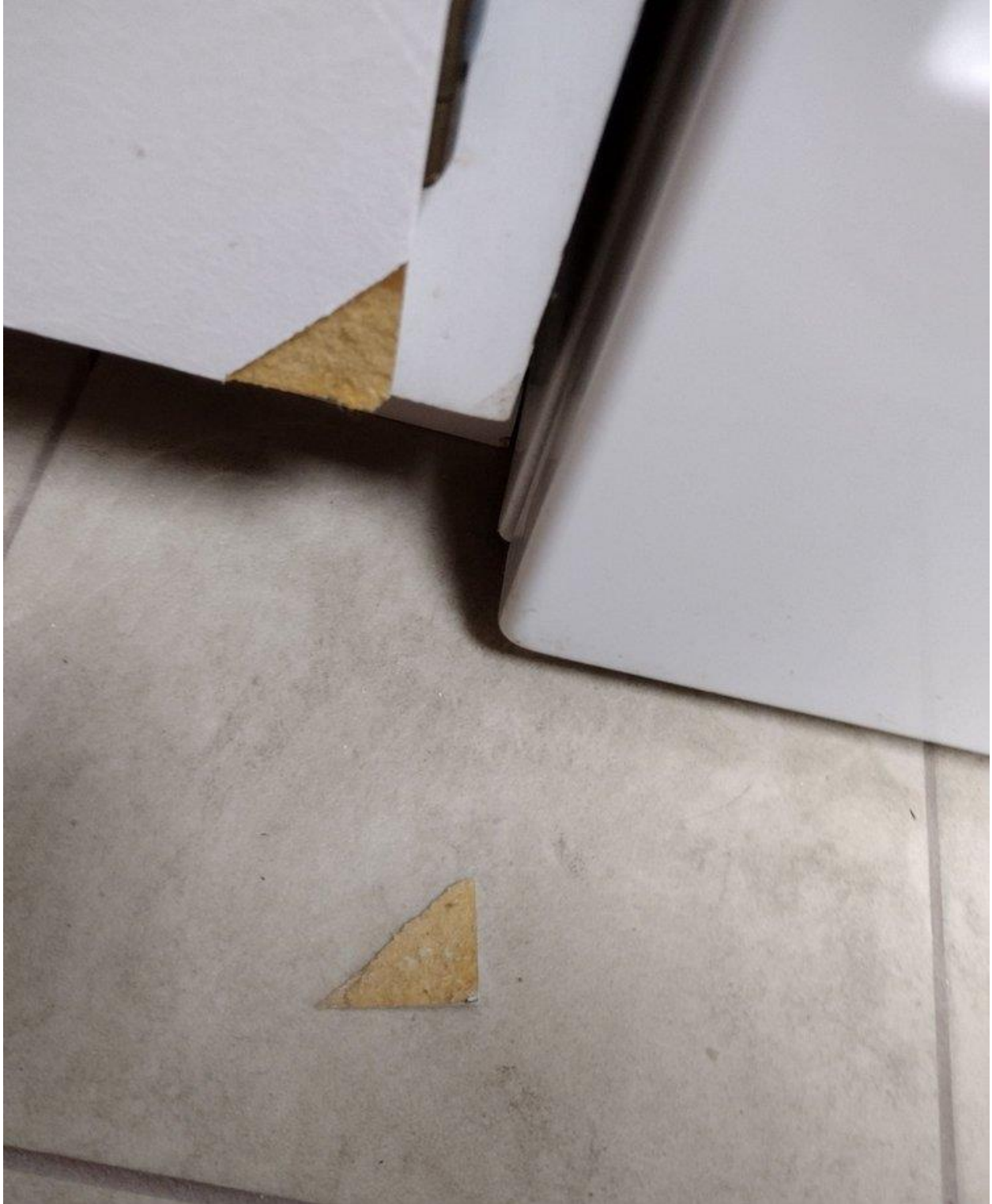
Broken kitchen cabinet, Photo 2.
