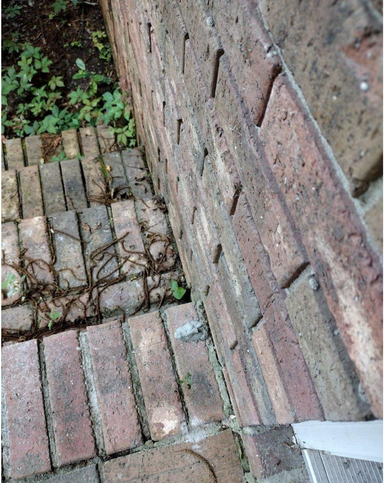
Thinset on brick porch, Photo 3. Big globs of thinset on the porch.
